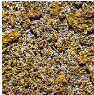
Rust Grade D
